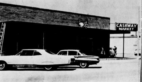
NEW FRONT--White's Cashway Grocery is getting a new front and an awning. This shows the work under way. (Journal Photo)
