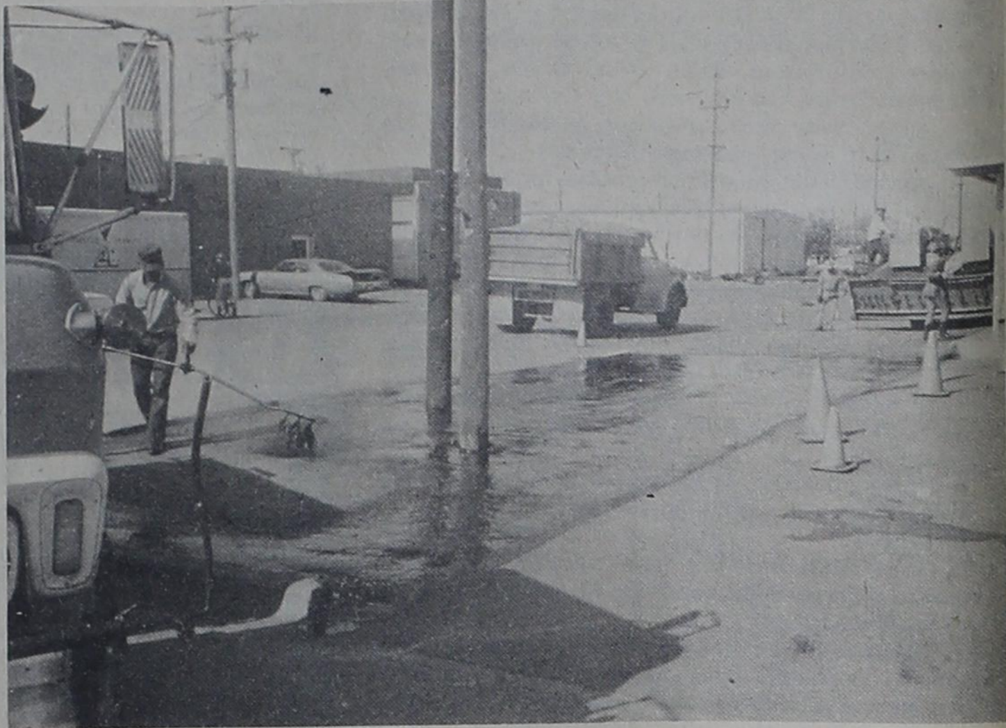
SPRING CLEANING is underway at the M-System Super Market as the parking area takes on a new look. New paving is being done by Coltharp Construction Company of Seymour. The 'new look' will certainly be appreciated by the store's customers.
