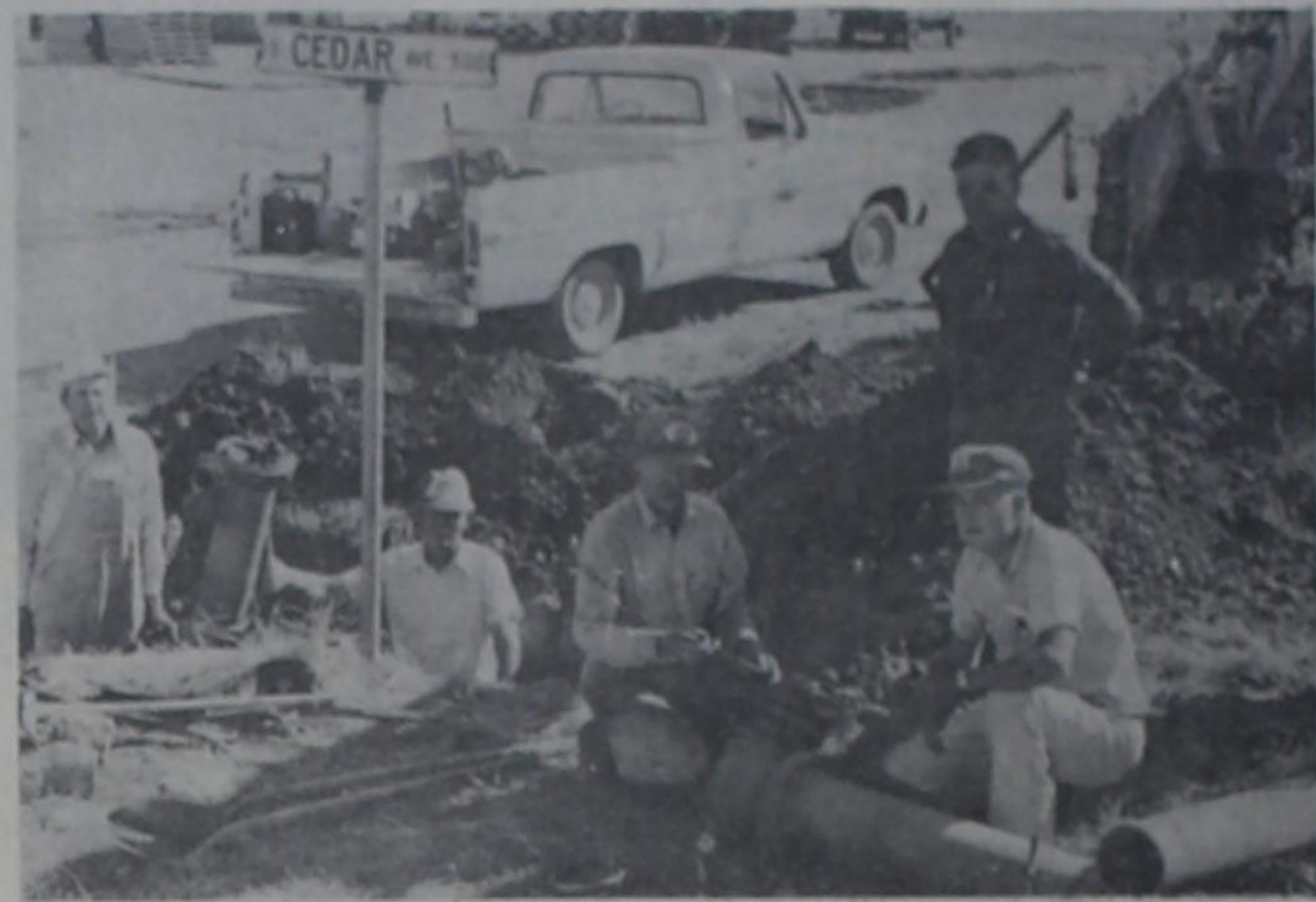
MAKING REPAIRS: Workmen for the City of Munday are shown installing a new water valve and fire hydrant near Abell Ag Co. recently as work continues on a state approved water system for Munday.
