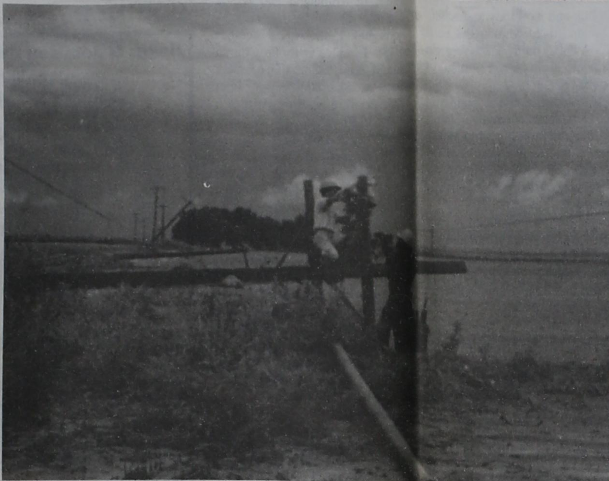
WITH THREATENING CLOUDS IN THE BACKGROUND, B-K Electric crews work to repair a downed line west of town following a storm that wreaked havoc in the area Thursday. Some outlying areas were without electricity for hours after the fast-building storm surprised many, with lots of hail, wind and rain.
