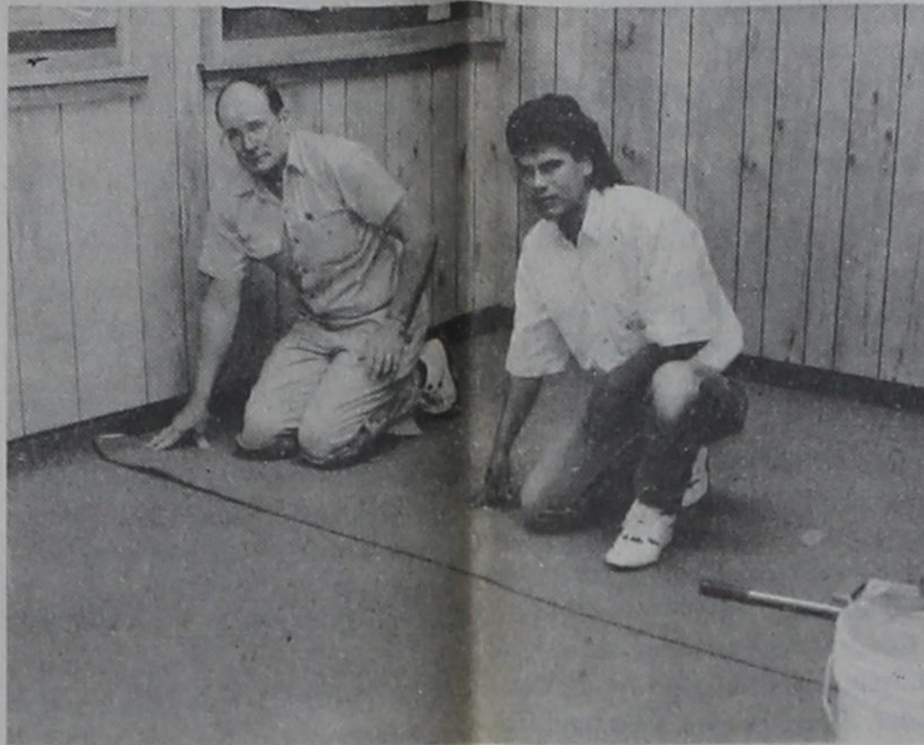
CHARLES YOST AND HIS HELPER, Noe Rosales, were caught by the photographer as they installed new carpet in one of the many classrooms in the elementary school that were flooded by broken water lines during the Christmas holidays.
