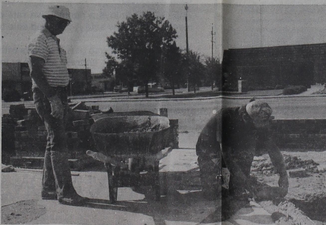
BRICKLAYING IS A DEMANDING ART, but Jimmy Urbanczyk (kneeling) makes it look easy. Jimmy, assisted by his father-in-law, Bobby Hutchinson, is building the low-profile brick wall in front of the Downtown Park, as well as constructing planting areas. When completed the area will serve a multitude of community activities. Plans are to have the area ready in time for the Munday school homecoming in October.
