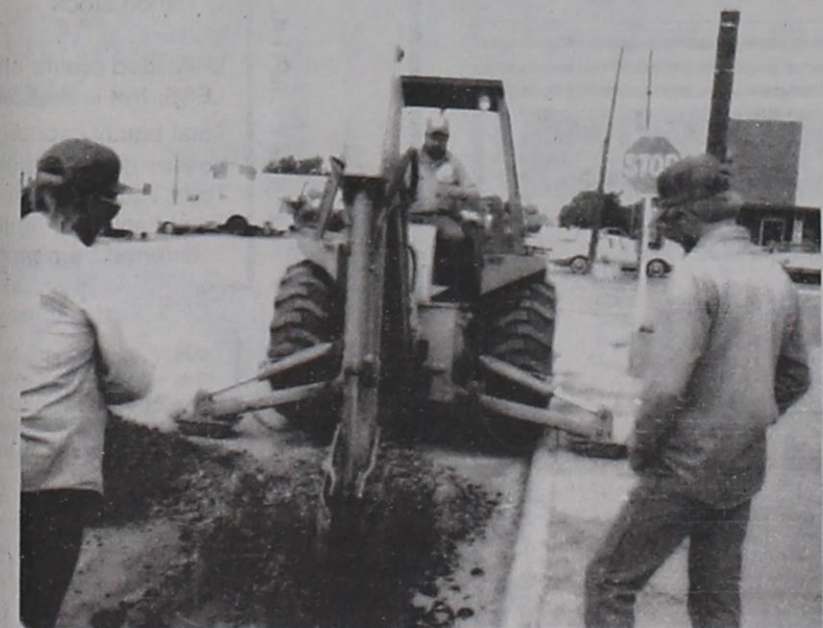
LONE STAR GAS EMPLOYEES searched three long and hard days for a gas leak. They finally located and repaired the leak on Friday. Workmen are pictured digging one of their holes in front of The Munday Courier office.
