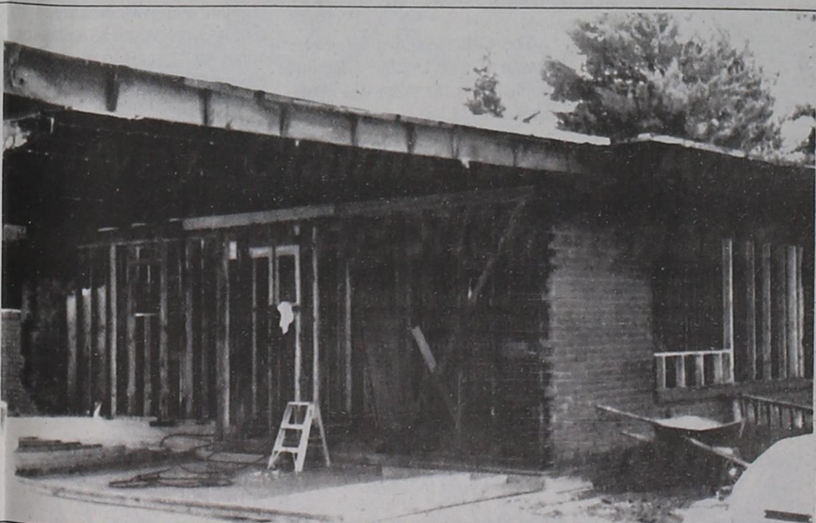
CONSTRUCTION IS UNDERWAY to repair the damage caused by a fire on May 21 at Michels Corner Inn. The office, lobby, kitchen and living area were destroyed in the early afternoon blaze. Business went on as usual, though, as they made one of the guest rooms into an office for the time being. The motel is owned by Collis and Ernestine Michels of Munday.
