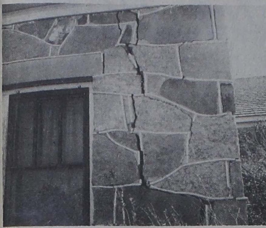
CRACKED WALLS Often results from building on clayey soil that shifts by becoming wet, then dry, at intervals.
