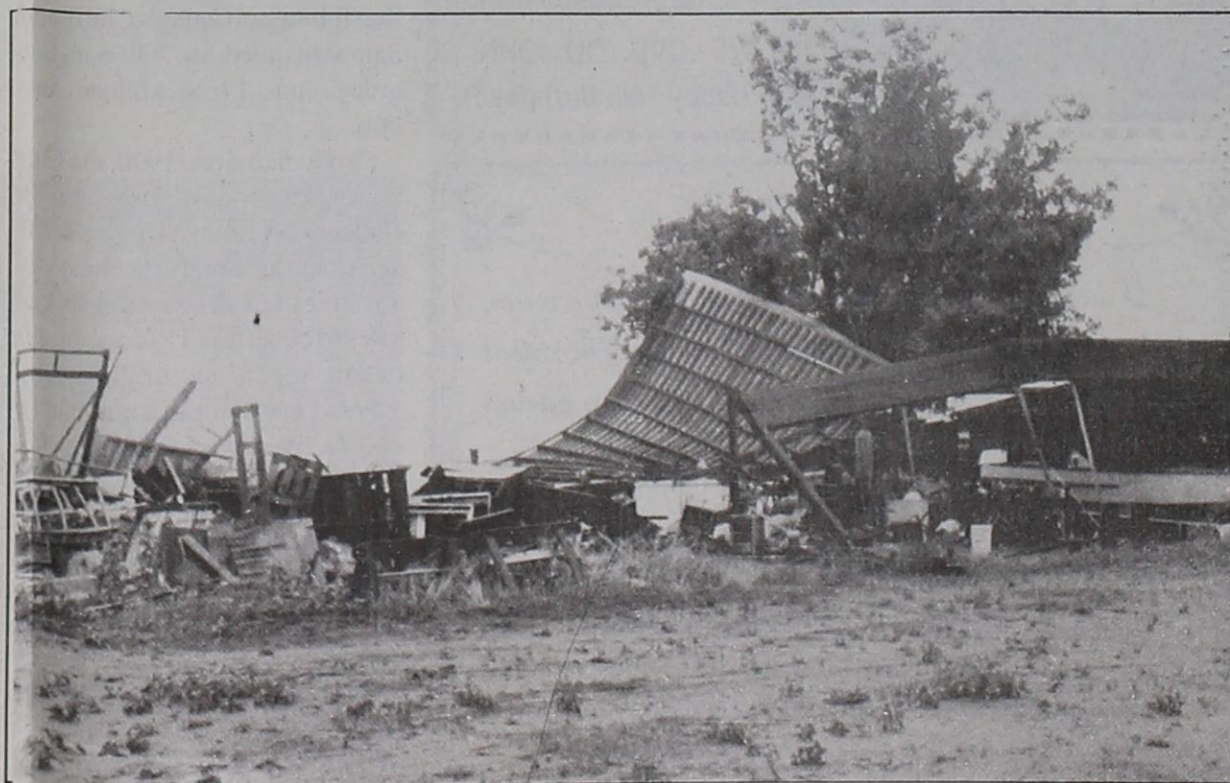
WINDS DESCRIBED AS STRONG AS A cyclone paraded near the Sunset community about noon June 9 and destroyed the farm shed of A.C. "Brownie" and Lena Tackitt. The shed held mostly tools and used lumber, but a pickup and motor boat parked in the center of the long shed escaped with just scratches. Winds reached as high as 70 mph in the first of two storms that day.
