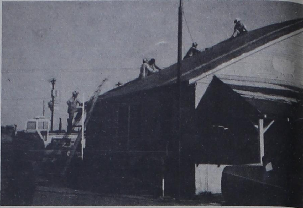
"A NEW HAT" for the office of Munday Gin and Seed was on the agenda of the directors and members of this organization. Instead of hiring the new roof put on, the men joined together and completed the job themselves.
