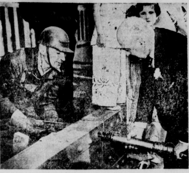
The last rivet was recently driven in the Golden Gate bridge at San Francisco. With many notables witnessing the ceremonies, a crew of iron-battered riveters drove a golden rivet into the span, signaling completion of the structural steel work.
