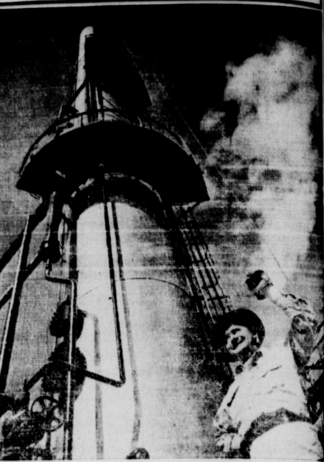
MILLIONS MORE GALLONS of 100-octane aviation gasoline for Uncle Sam's super bombers blasting Japan's war industries will flow from this huge plant recently completed by The Texas Company on the Pacific Coast.
