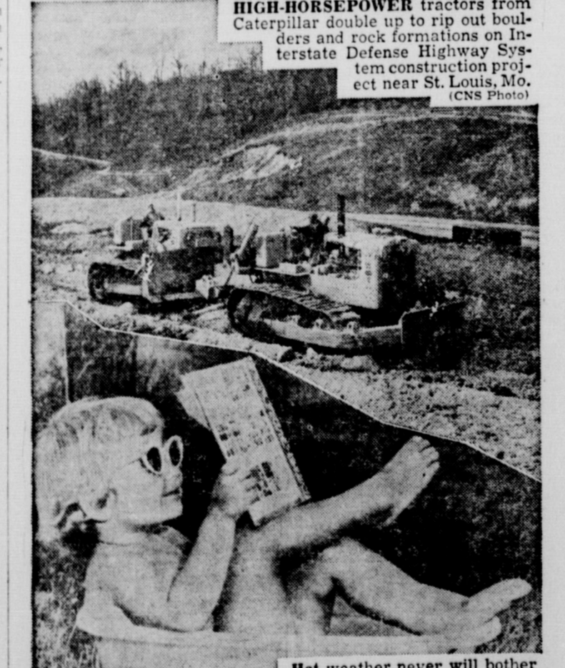
HIGH-HORSEPOWER tractors from Caterpillar double up to rip out boulders and rock formations on Interstate Defense Highway System construction project near St. Louis, Mo. (CNS Photo)
