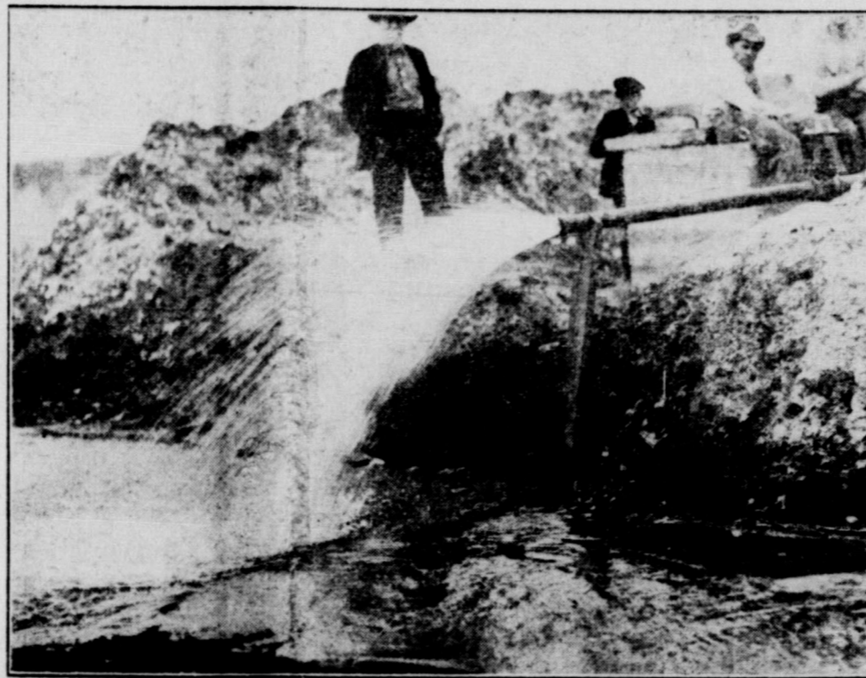
Pumping Water at the City Well Near Crowell to Keep It Out of the Way Until Big Reservoir Could Be Completed. Photo Made by Clifton Studio.
