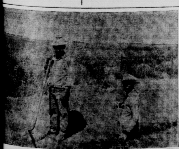
WORKING ON WATER SYSTEM —Shown above are Willie Garza and Rual Brown, both of Crowell, as they shovel dirt on the water line from the wells to Thalia. A thin layer of dirt was placed on the pipe, and the trench will not be completely filled until the line is checked for leaks.
