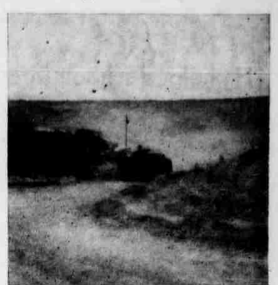
Big earth mover roars up road across front face of White River dam for another load of rock for rip rap. Note rip rap face of dam in background.
