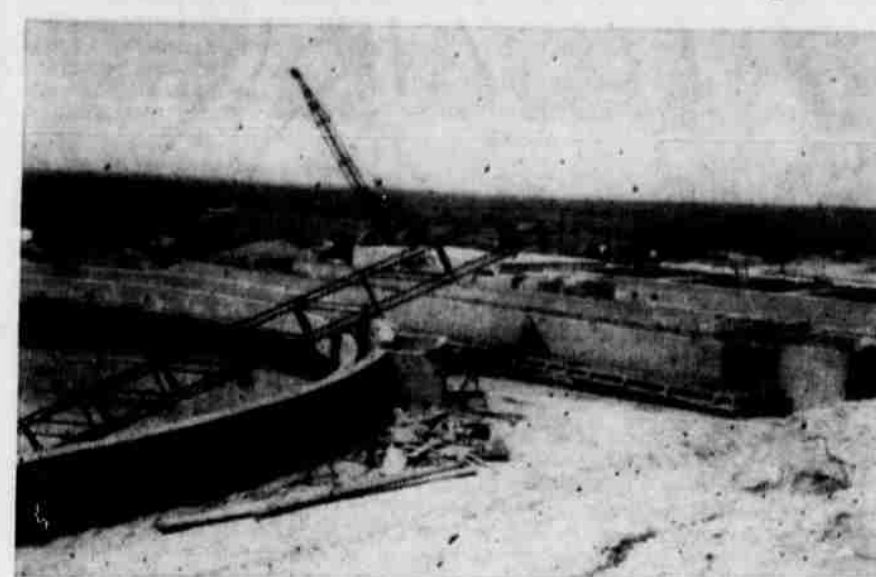
This view shows part of filtration plant clarifier to left, the flocculator in middle where lime is added, and a portion of the four filters in a line in structure at right which provide final treatment of lake water.
