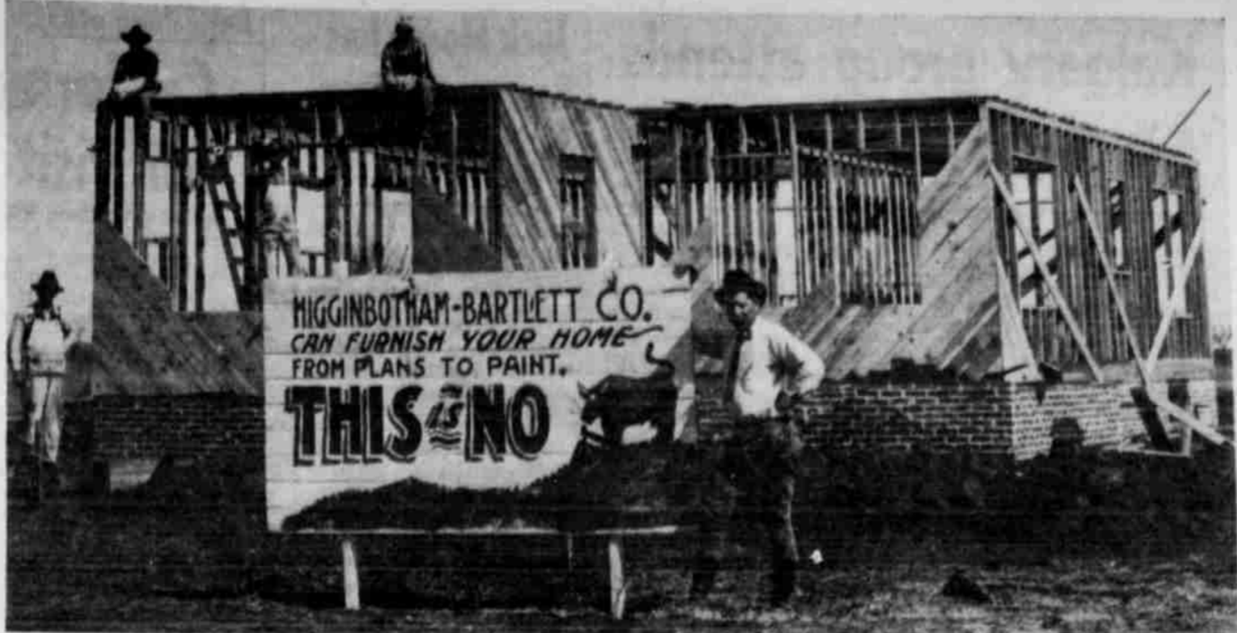
Shown above is a 1924 picture of Higginbotham-Bartlett Co. workmen building a new Post residence at 516 West 12th Street, the home of Dr. L. J. Morrison today. The man in the boots and pipe leaning on the sign is Tom Bouchier, manager of the firm's yard here.
