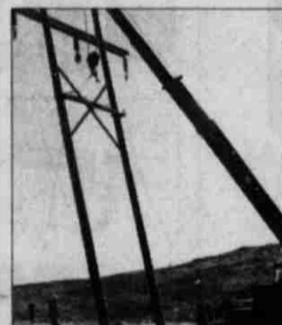
"We're putting in a new 115,000 volt line . . . gives us another feed to back up our dependability . . ."
