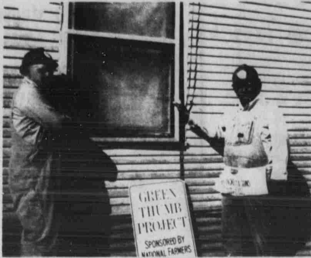
WINTERIZING HOMES — Garza County's industrious Green Thumb crew is busy winterizing and repairing homes over the county of those on fixed incomes who cannot afford such repairs. Shown above, left to right, Green Thumbers R. L. Reeves and Juventino Sanchez busy on a local home. — (Staff Photo)
