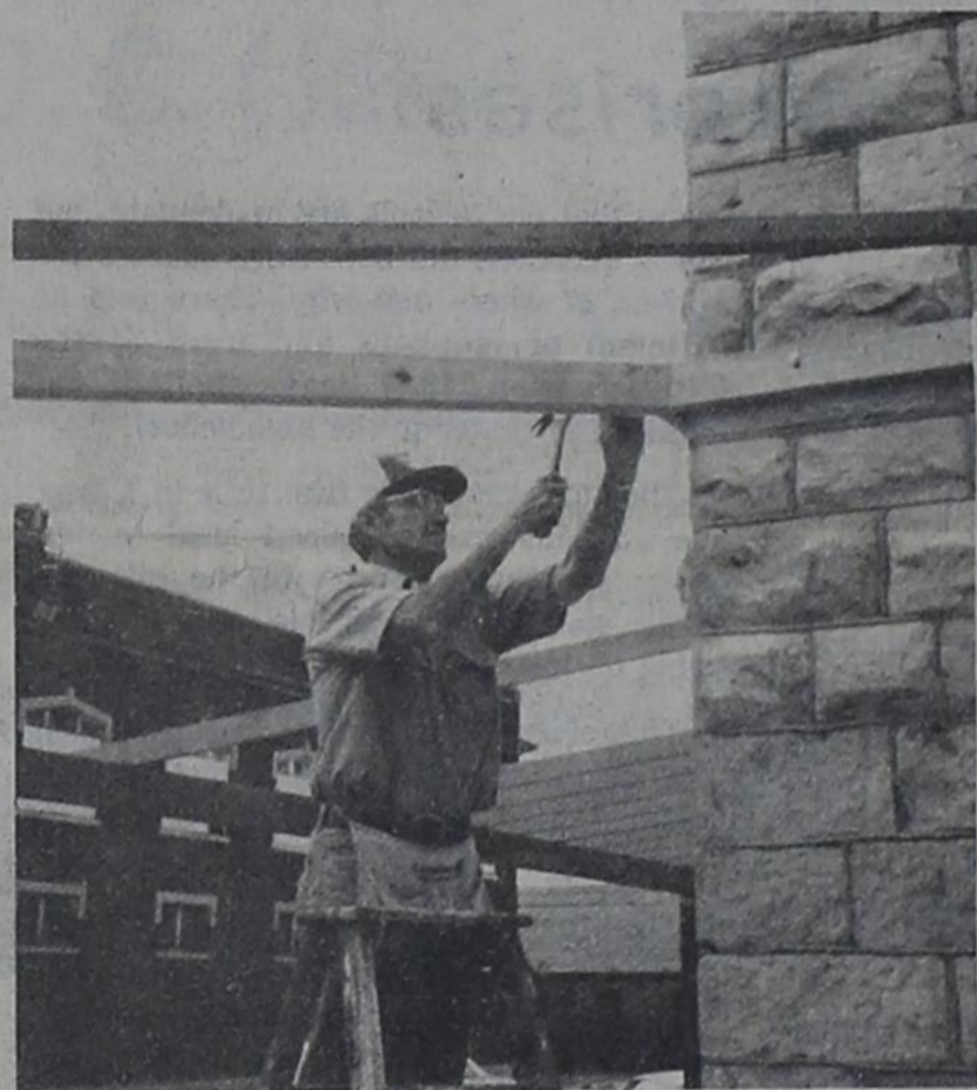
ALGERITA'S AWNING COMPLETE — The wooden awning over the sidewalk has been completed for the historic Algerita hotel with the shingling of it this week. The restored exterior of the hotel is shown in the upper picture with its new awning extending across the front and halfway down the side. In the bottom picture, David Newby is shown as he began work on the awning three weeks ago. — (Staff Photo)
