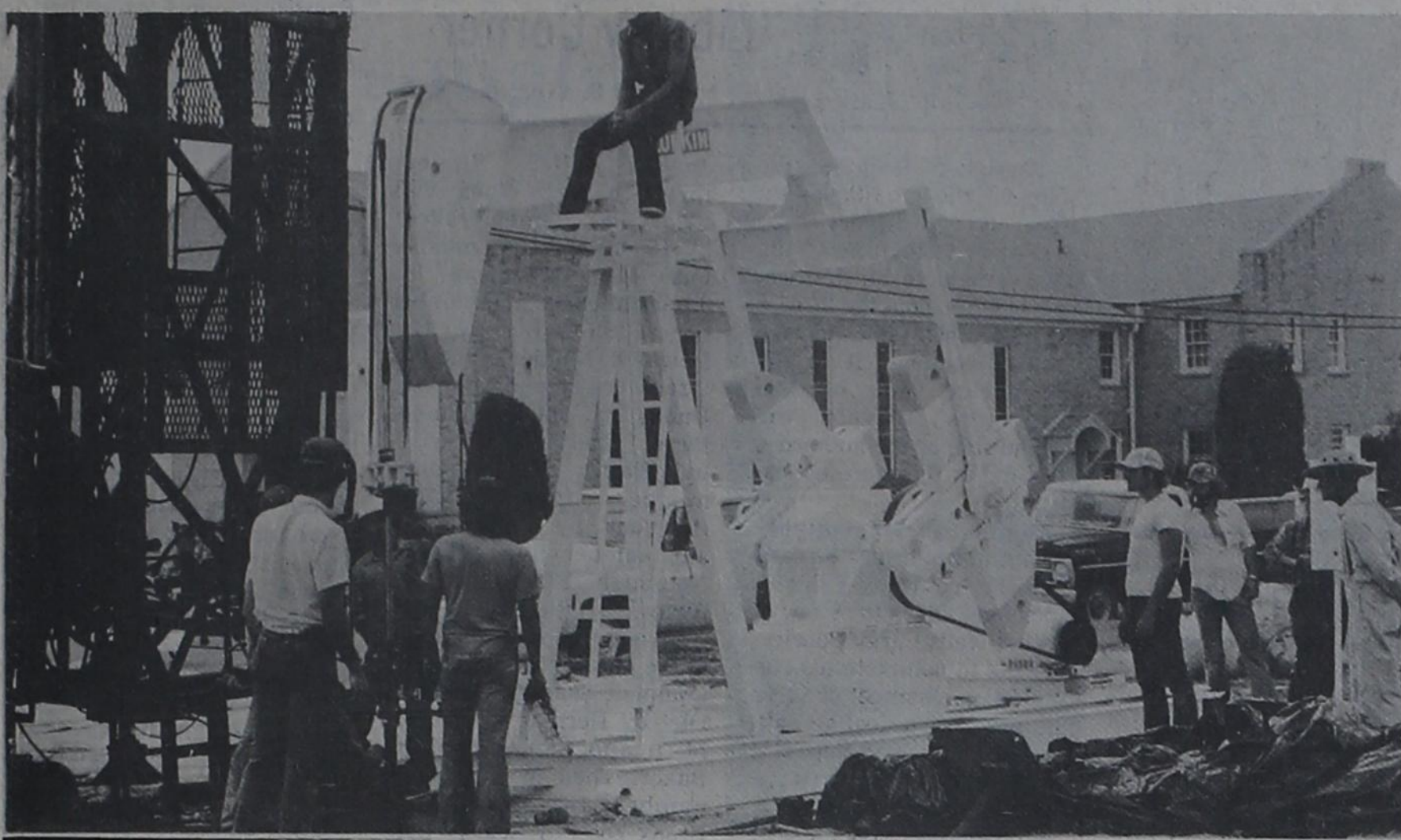
POST'S NEW 'SHOW WELL' — Looking almost like a white ghost, the white pumping unit with gold trim was installed on the new well behind the Garza courthouse Friday. Shown around the
