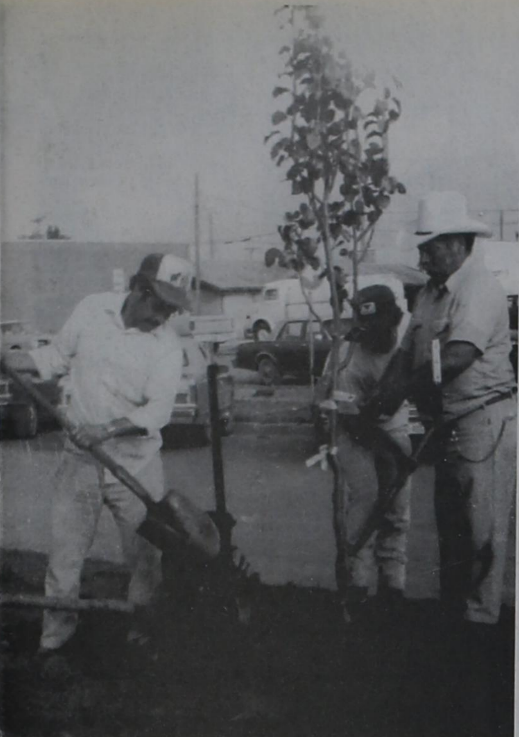
NEW TREES FOR MAIN STREET were planted last week by Walls Green Enterprises, contractor for the landscaping project. Planting the container grown Bradford Pears and Red Oaks were (left to right) Jose Olivares, Manuel Alcalá and Don Mims, all of Dallas.
