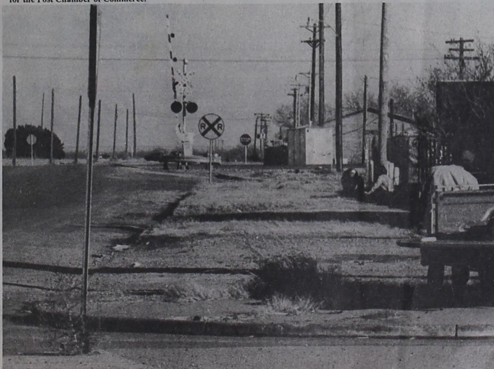
WORK BEGAN this week on reconstruction of East 15th Street between U.S. Hwy 84 and SH 207. Part of the work will include raising of the railroad tracks and installation of new signals.
