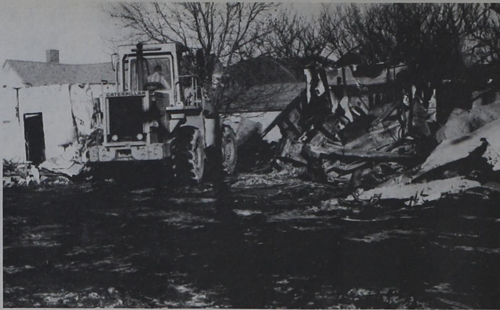
FINAL CLEANUP - The last scraps of what was once a Post landmark are hauled away by H & M Construction Co. crews following the fire that destroyed Jackson's Cafe on U.S. Hwy 84.
