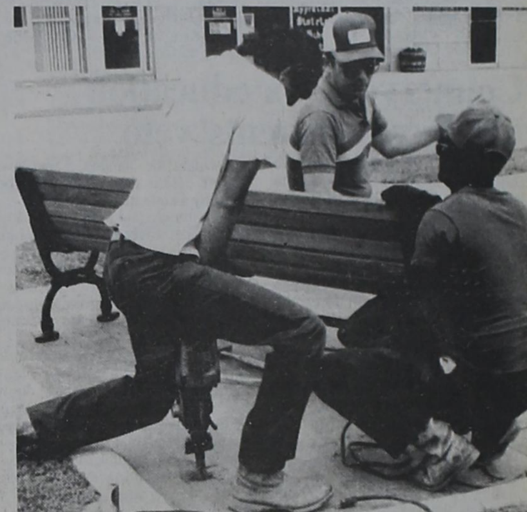
CITY CREWS were busy last week installing the mahogany benches in the plaza areas of the newly complete landscaping on East Main Street. Working on installing the benches are (left to right) Frank Flores, Delbert Rudd and Owen Gilbert. The benches have been purchased through private donations.
