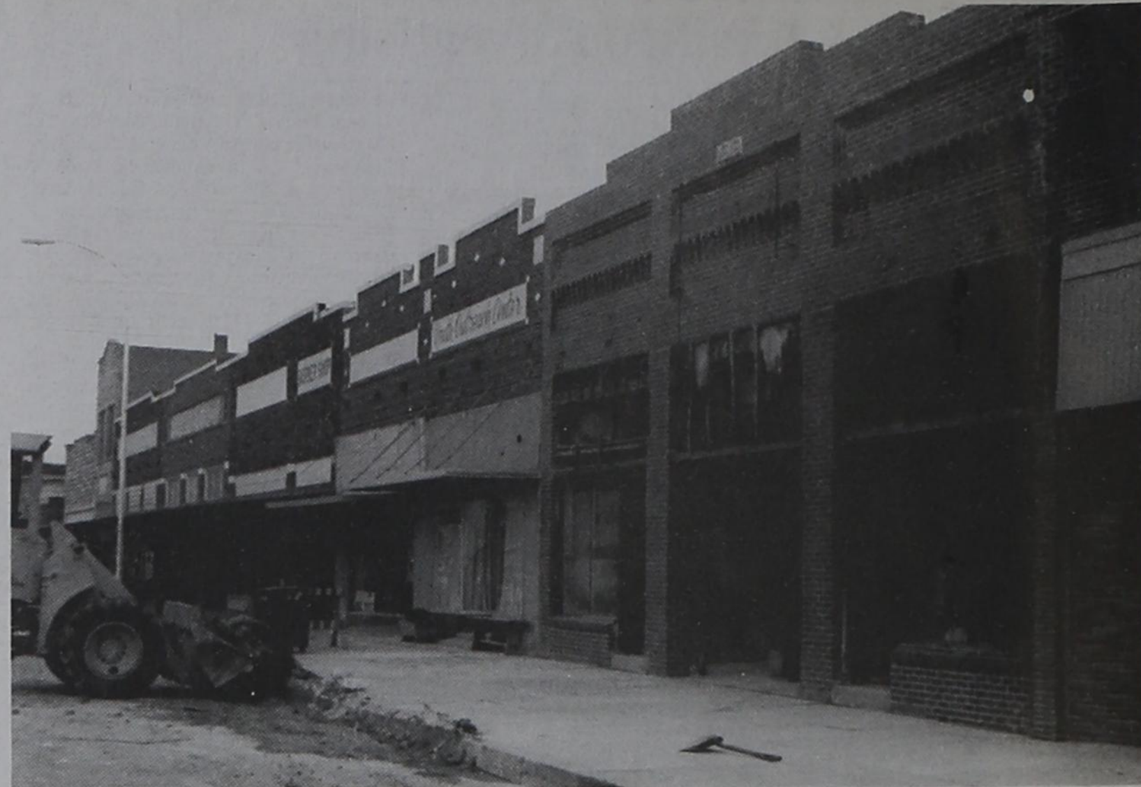
WOW WHAT A DIFFERENCE - Brick work on the front of the Garza Theatre was completed this week, and work on restoring the front of the building is beginning to really show the signs. Garza Theatre board member A.C. Cash has been supervising the project, which is bringing more and more attention to Post.
