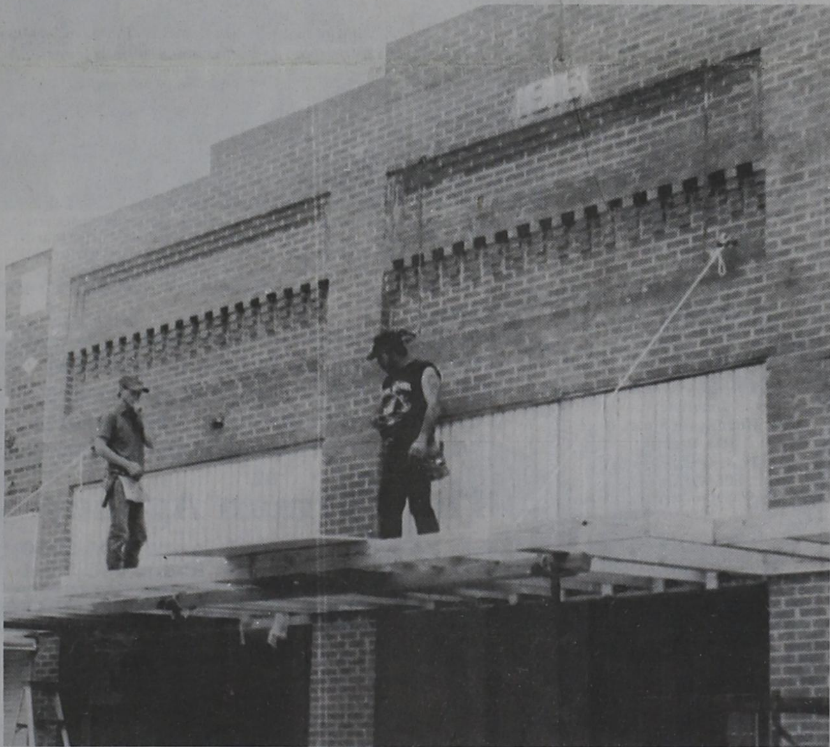
WORK CONTINUES at the Garza Theatre as the front of the building now gets a fresh awning, which was appreciated last weekend by theatre patrons.
