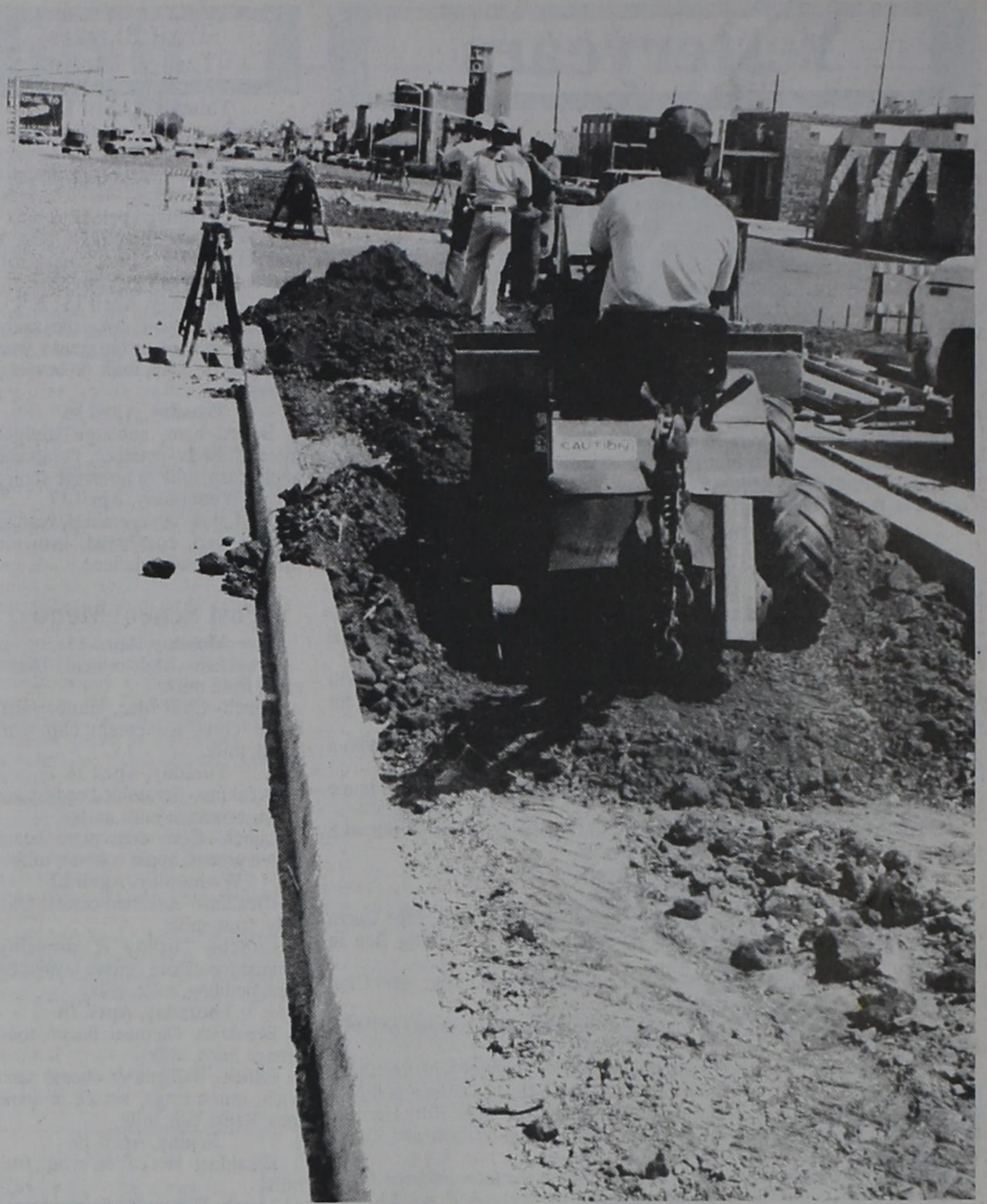
EAST MAIN STREET landscaping begins to take shape as construction crews level dirt in preparation for grass and trees. The project, which is funded through private donations, has been contracted with Bo Jackson.
