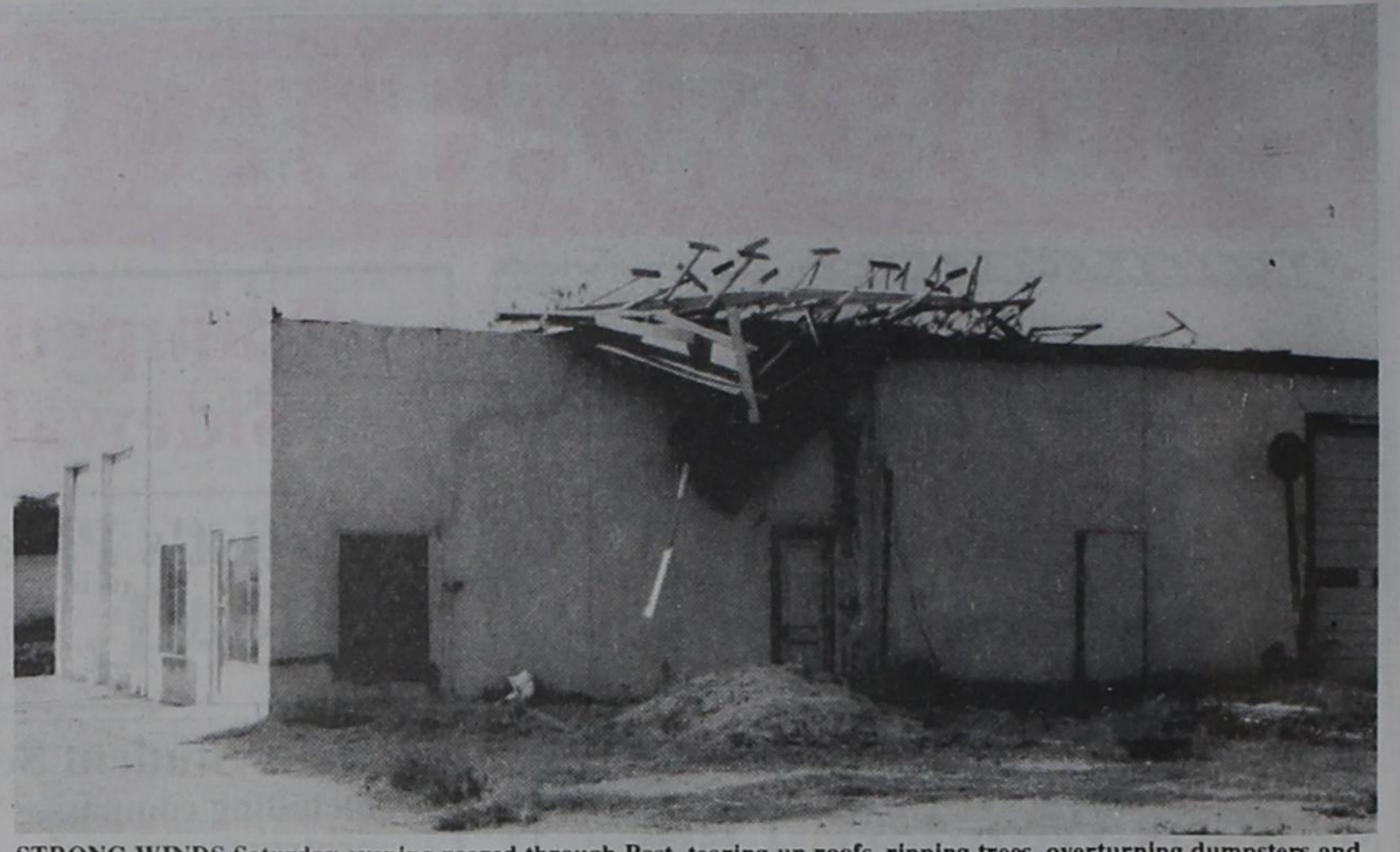
STRONG WINDS Saturday evening roared through Post, tearing up roofs, ripping trees, overturning dumpsters and other damages. The old C.R. Wilson service station on South Broadway took a big hit when the new roof was completely smashed.
