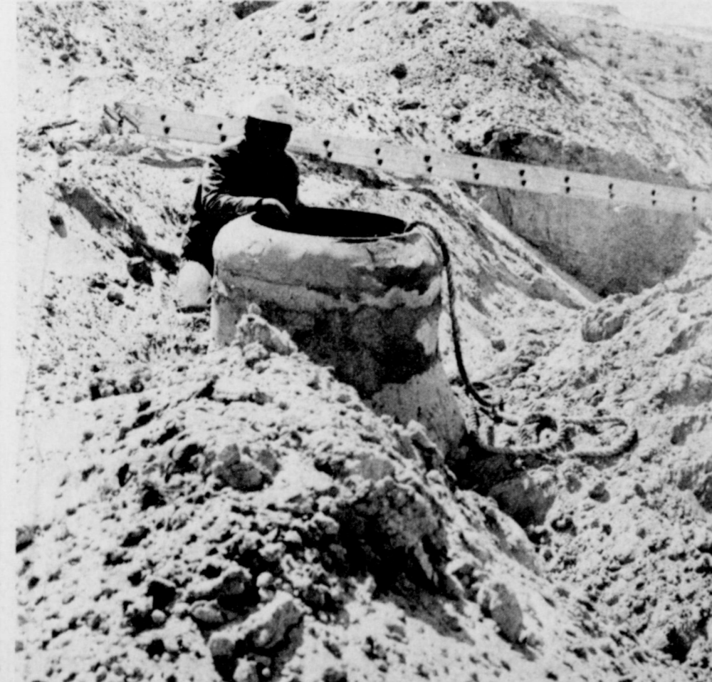
INSTALLING MANHOLES--This workman talks to a fellow workman at the bottom of a manhole under installation in the new Parkridge Addition in southwest Muleshoe. More than 20 lots will be available in the initial phase of the new addition for construction.
