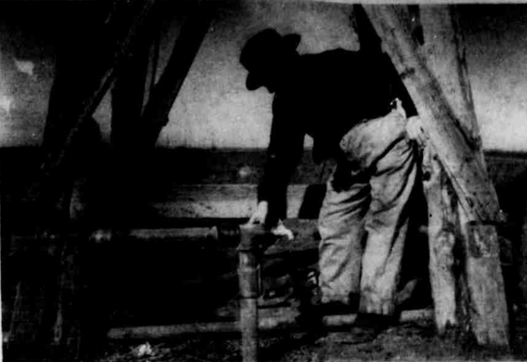
FROM THE OLD TO THE NEW—S. D. Lofton is shown shutting off one of the valves which controls the flow of water in his unique irrigation system, which includes one irrigation well and two windmill wells at which small electric pumps have been installed. Lofton irrigates 30 acres with the system, which also supplies water for household and other needs. —(Staff Photo.)
