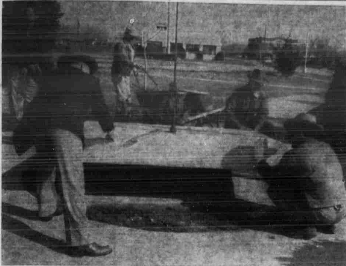
STATUE BASE GOES DOWN — The base for the statue of C. W. Post, to be unveiled April 5, is being placed in the memorial circle on the courthouse lawn. Directing the operations is Jim Collier (upper right) of the South Plains Monument Company in Lubbock. The pedestal and veiled statue followed. — (Staff Photo)
