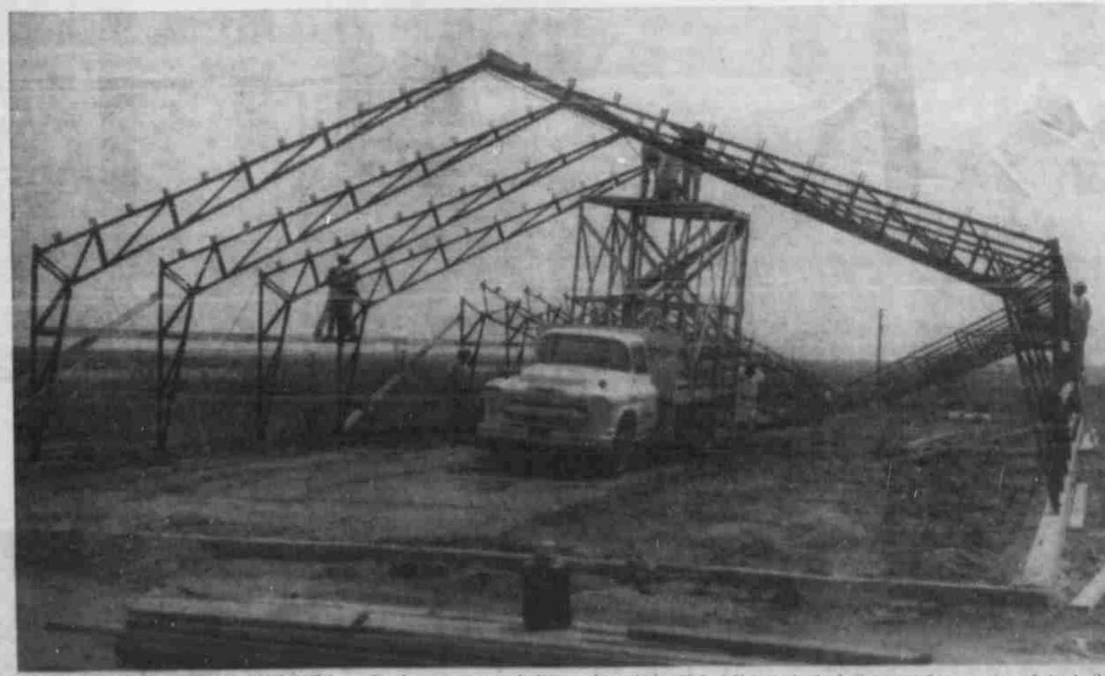
STEEL GOES UP ON 4-H BUILDING — Steel girders are being erected on the all-metal 4-H Club building under construction on the south side of the city-county park. The building, a county-wide 4-H project, is to be 44 by 60 feet with concrete floor. Adjoining it will
