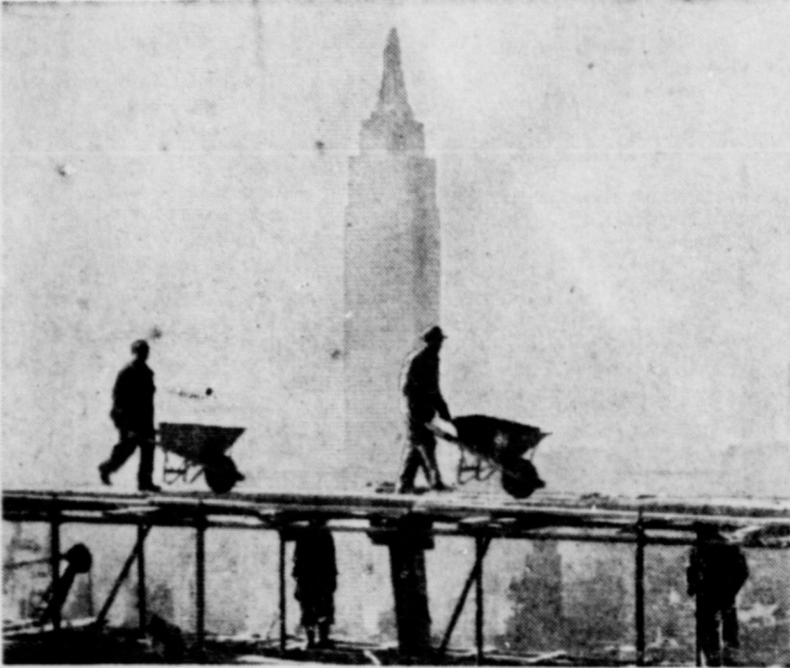
MONUMENT TO PEACE . . . This new view of progress being made in construction of the United Nations world headquarters in New York City shows workmen carting their wheelbarrows of cement on the 39th floor, in the shadow of New York's tallest skyscraper, the Empire State building.
