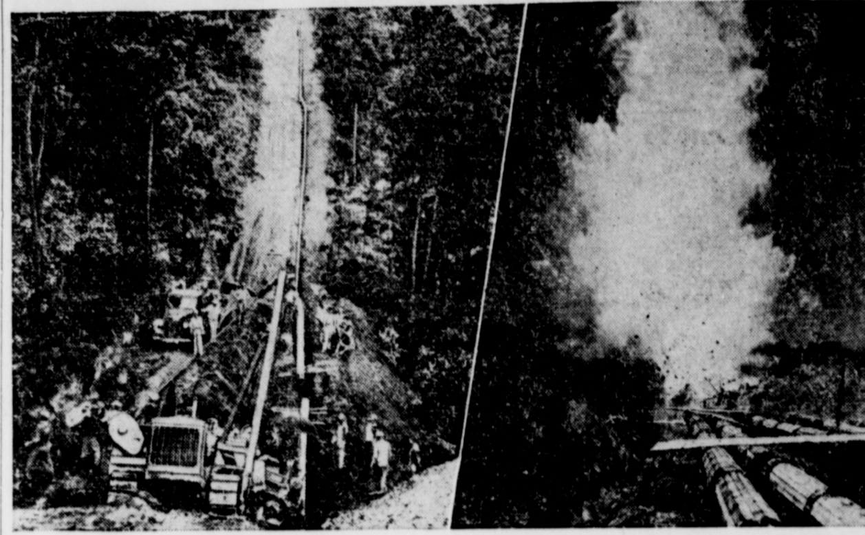
When a petroleum pipe line is being built to supply war industries with the precious fluid, nothing stops the pipe line gangs. Right: A rock ditch being blasted at a river crossing somewhere in the Carolinas. Left: A gang prepares to bend a 12-inch pipe in the mountain area of Alabama. Bending the pipe to conform with the terrain is tough work. The completed Plantation Pipe line, from Baton Rouge, La., to Bremen, Ga., and Greensboro, N. C., has some 1,200 miles of pipe.
