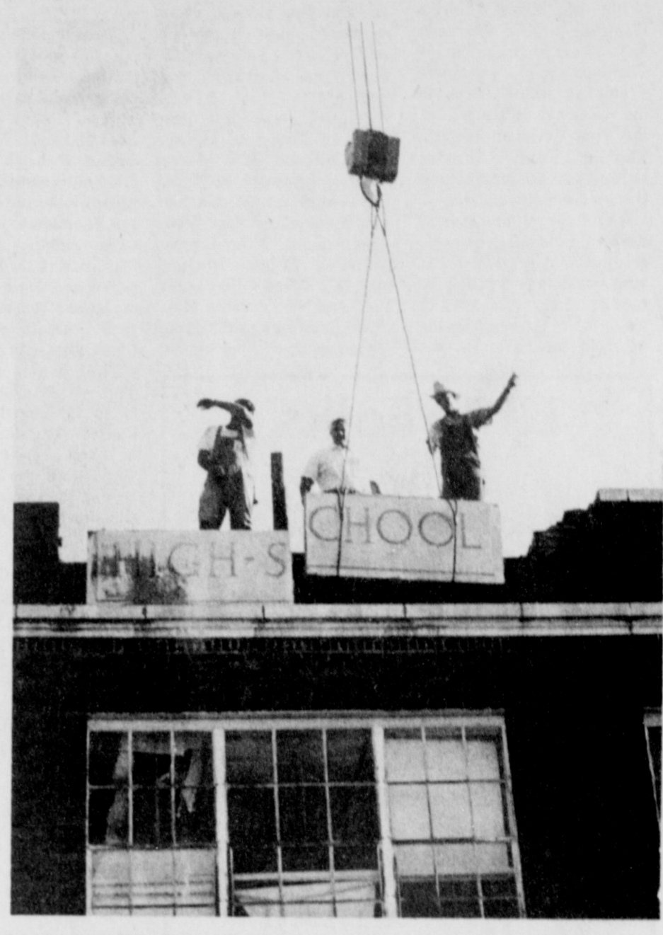
NAME SAVING -School officials and a demolition crew made an effort to save the name stone which crowned the old W.F. George High School here. With the aid of a mammoth crane supplied by Barbour Trucking Co. the landmark successfully was removed in four sections. The task took about an hour.
