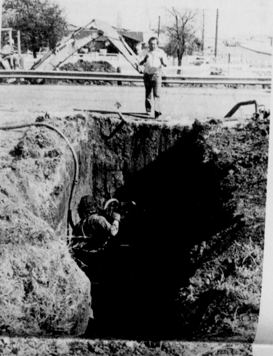
DIGGING FOR WATER? Nope, workmen were boring beneath Johnson Road this week as part of a project to lay telephone lines underground through the north side of Iowa Park. The effort is part of a 50-mile project to connect underground lines between Wichita Falls and Vernon, which eventually will connect the Dallas and Fort Worth area with Amarillo, all underground. The line will have 14,000 circuits. Eventually there will be no overhead lines along the route served by Southwestern Bell Telephone.
