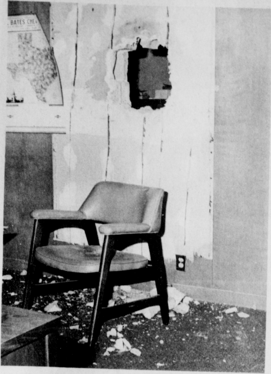
BURGLAR'S SMALL HOLE THROUGH VAULT WALL ... same hole used two years ago.
