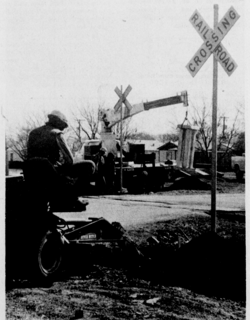
CROSSING GUARD - Workmen this week installed equipment for a railroad crossing guard on Jackson Street. It will be of the same design as the one on Johnson Road. The installation is jointly financed by Iowa Park, the railroad and federal funds.
