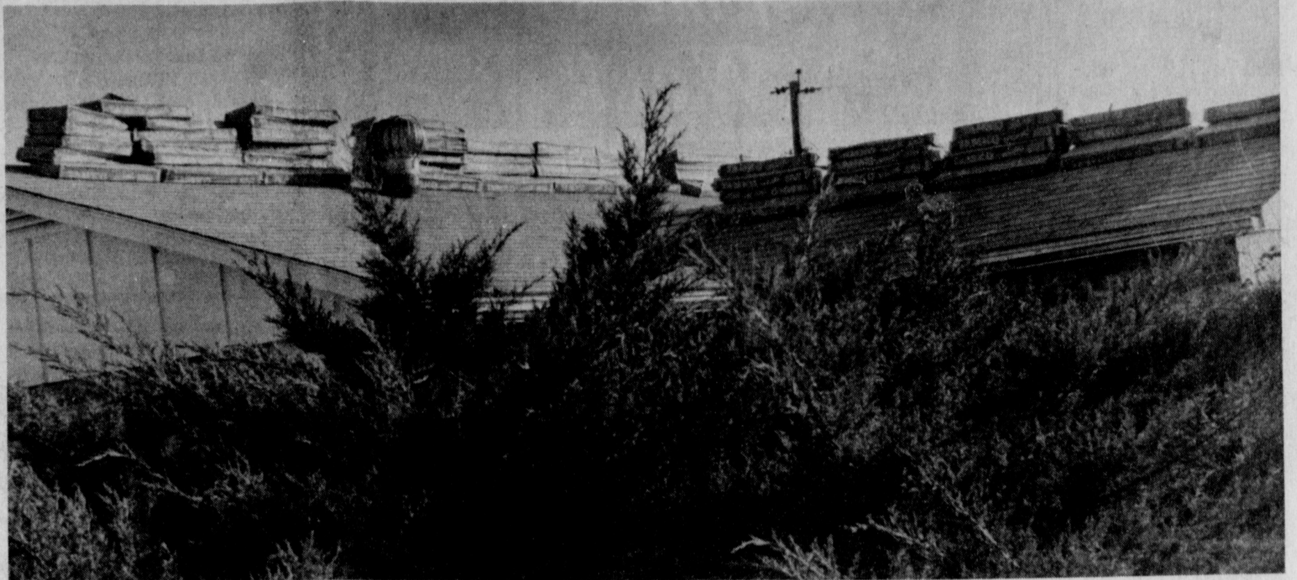
NEW IOWA PARK SKYLINE - As workmen begin repairing almost every roof in Iowa Park, the skyline is changing to the jagged appearance of bundled shingles awaiting the workers' attention. More than 1,000 home and business
