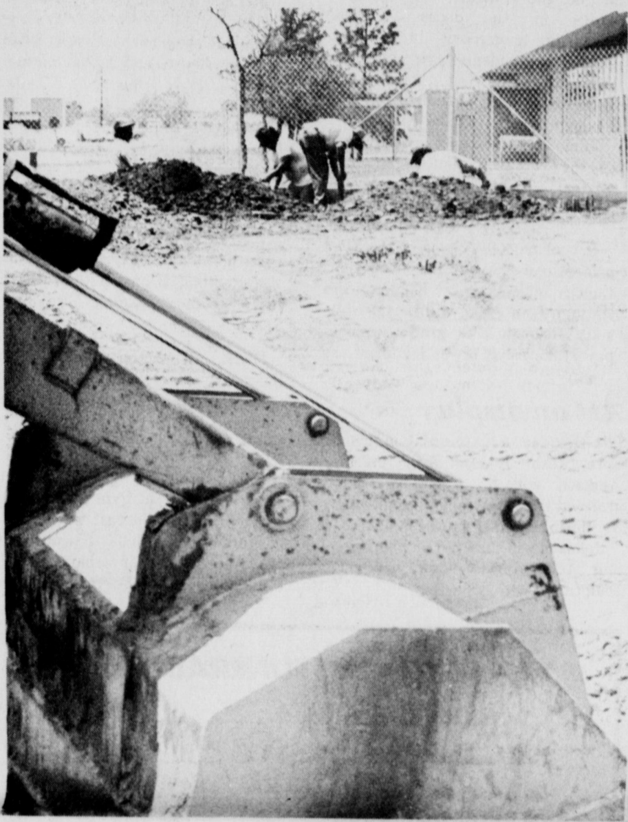
CONSTRUCTION BEGINS - Workers began this week with site preparation on the new music building at Bradford Elementary campus. The area has been fenced for the protection of students who will begin classes Monday.
