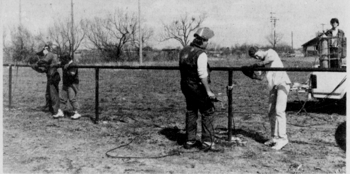
DOING THEIR PART - These five students, along with others in their Vocational Agriculture class at Iowa Park High School, made a major contribution to building the new Senior Little League Baseball field, located on West Highway behind Sonic Drive-In and Harvey's. Shown constructing a pipe fence are Will McCarthy, Mike Manry, Mike Thorne, Tommy Collins and Jim Shea. It was part of the Iowa Park Future Farmers of America Chapter's Building Our American Communities program, which received a $500 grant from the Texas Rural Communities.
