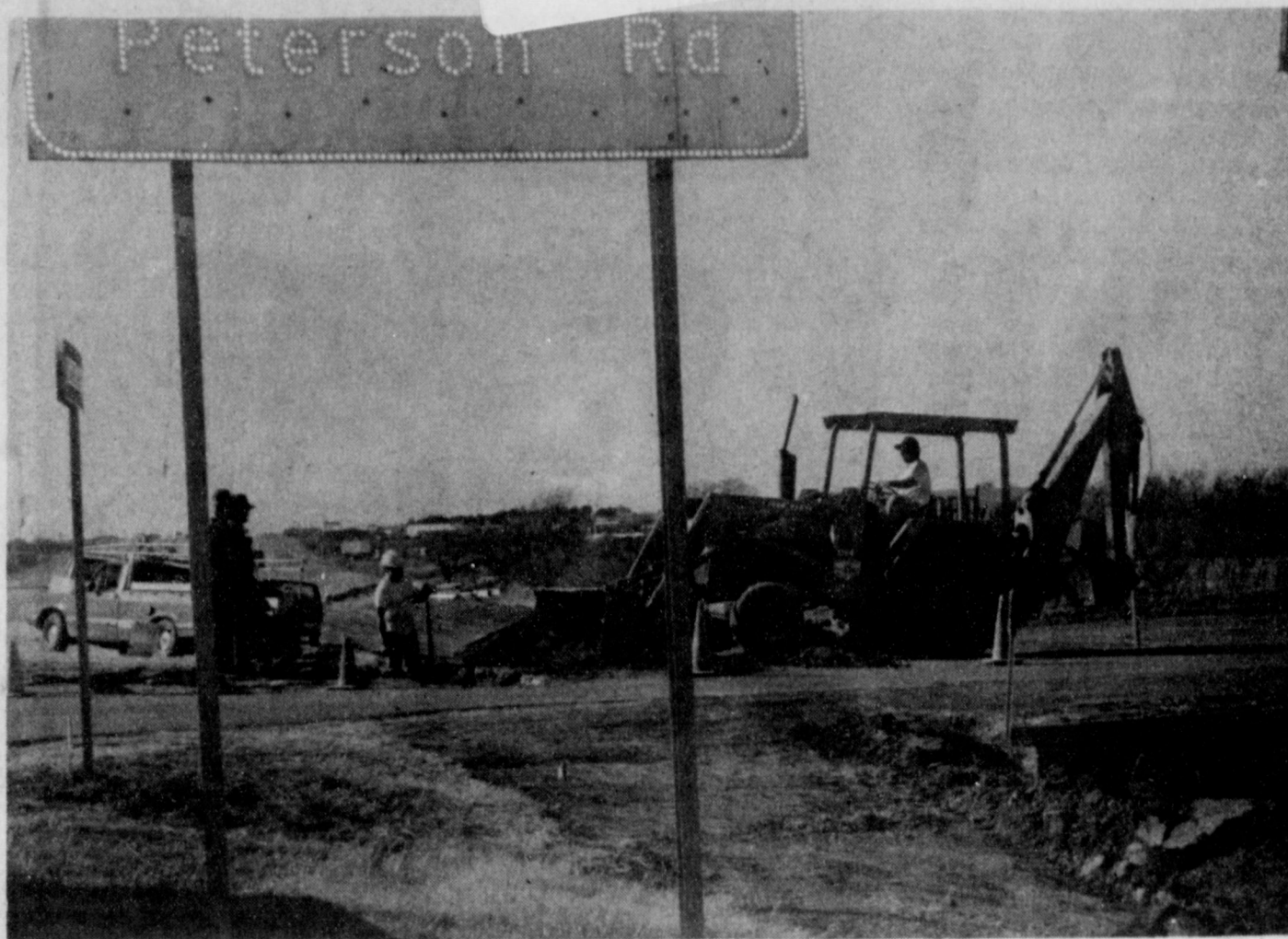
CONSTRUCTION UNDERWAY - Preparatory work for constructing a Peterson Road overpass at US 287, and an access road from there to Bell Road, is well underway.
