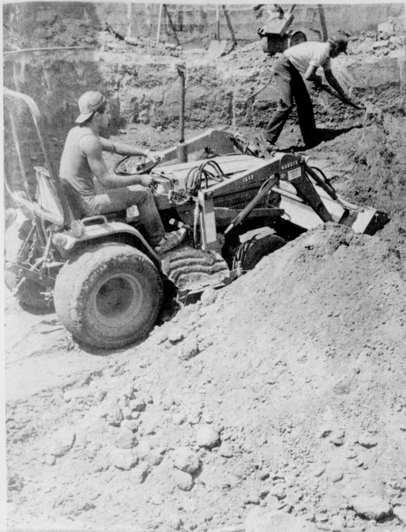
FILL-IN OPERATION - City employees this week filled and packed sand in three basement areas on the vacant lot west of city hall. The work is in preparation for construction of a new Chamber of Commerce office building.
