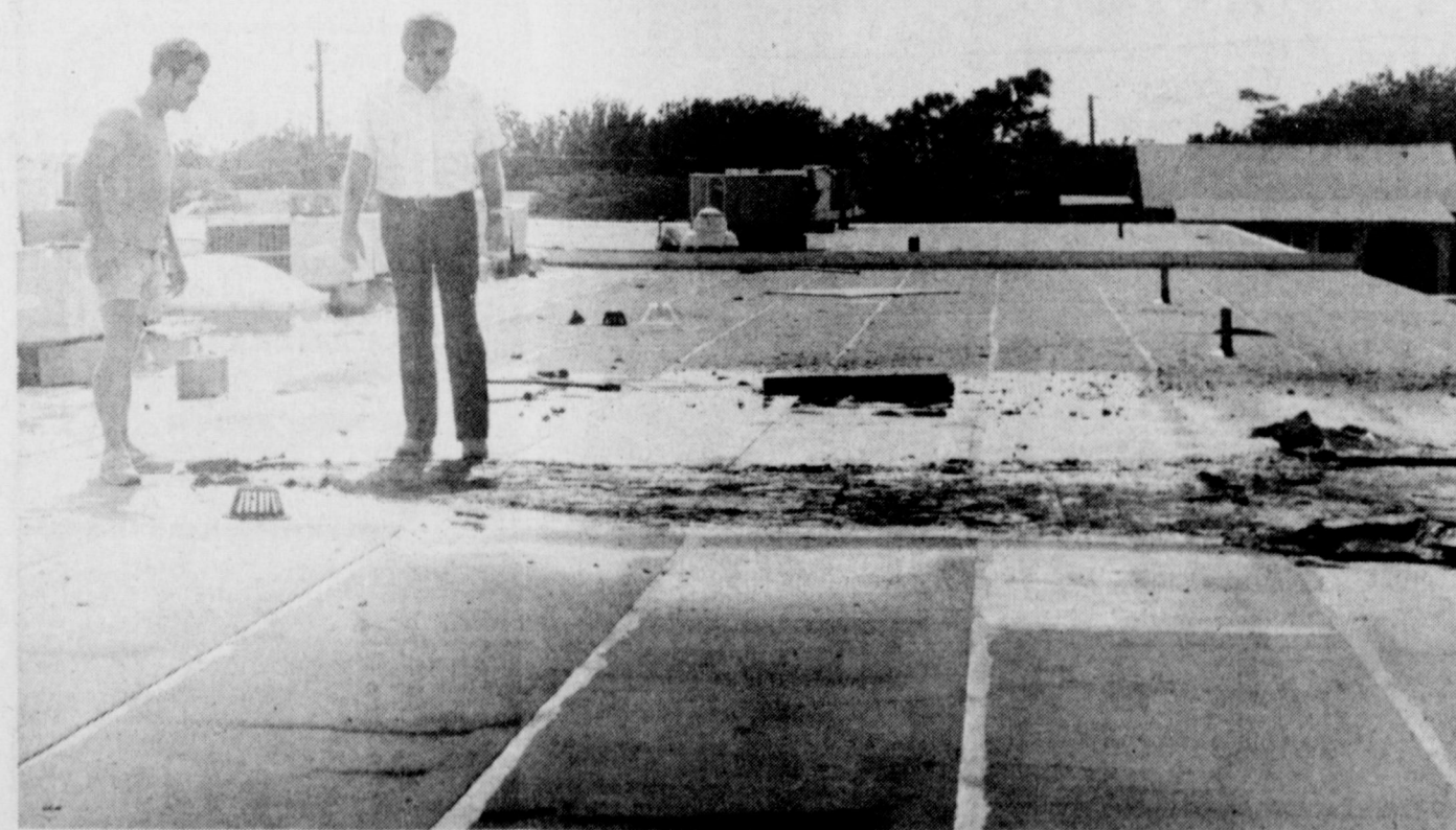
FIRE DAMAGE SURVEYED - Fireman Mark Wicks and Sonny Bates, city code enforcement officer, inspect damage fire did to the roof of Kidwell Elementary Thursday afternoon after a roofing crew quit for the day. An investigation is underway to determine the cause, but hot tar or a worker heating tar for the roofing project are suspected. A strong southerly wind that forced the blaze on its shortest course and quick response by volunteer firemen held damage to a minimum.
