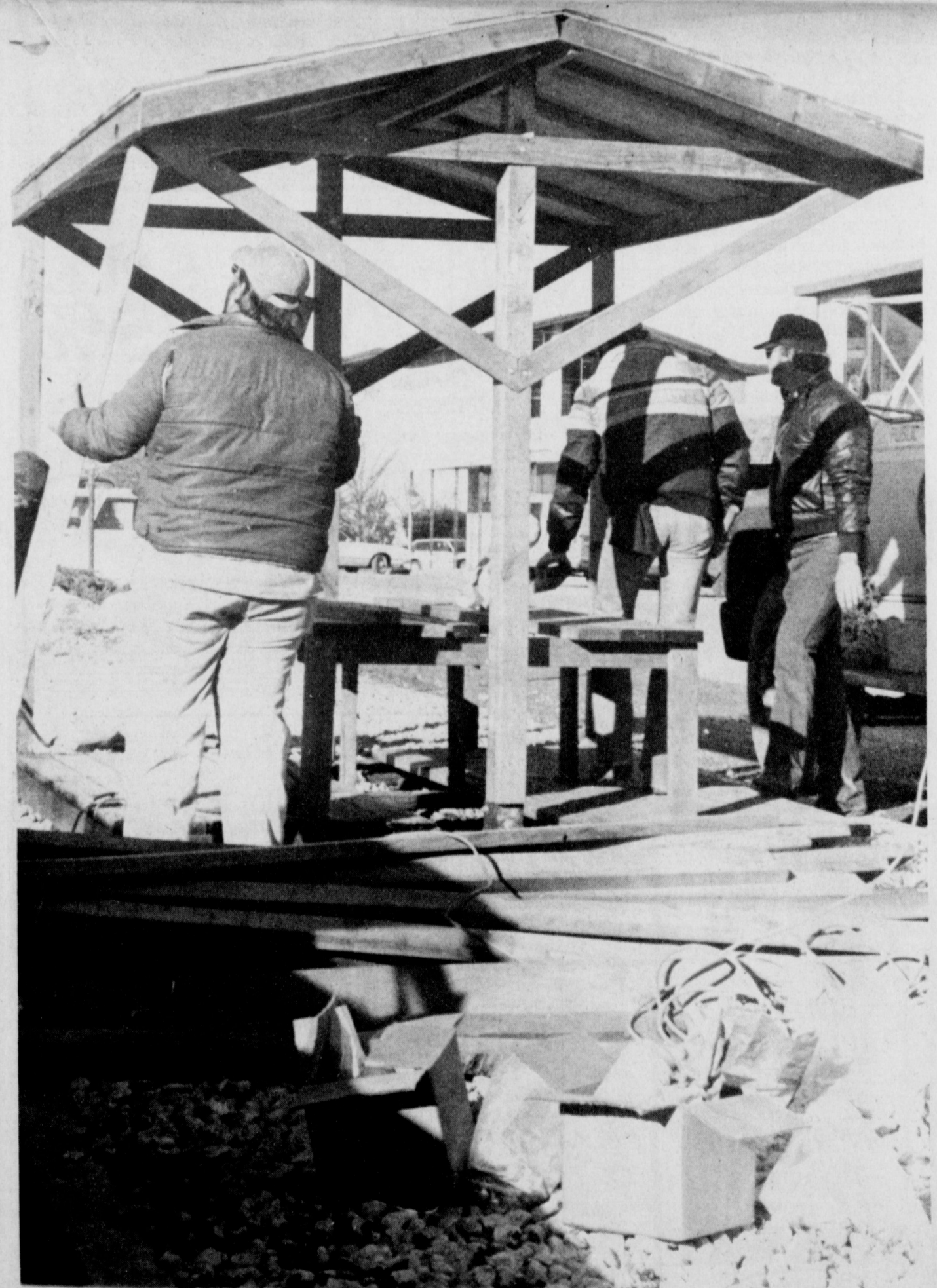
CITY WORKERS this week erected two covered bench rest areas in the median area of the 100 block of West Park. The redwood structures, which will have flowers planted nearby, are part of the business area improvement project begun last year, and were financed jointly by the Park Board and Independent American Savings.
