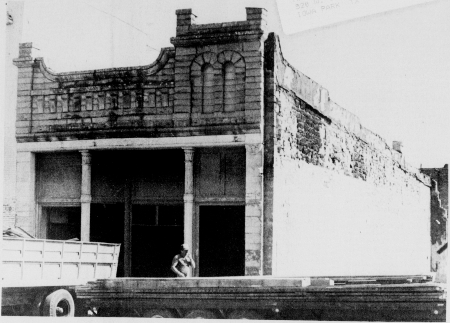
OLD BUILDING COMING DOWN - One of Iowa Park's oldest business building will no longer be, as workers began Tuesday tearing it to the ground. The 105 W. Park structure was condemned by the city because of its condition, and owner Stanley Williamson was instructed to repair it or tear it down. City inspectors discovered its old rock walls crumbling after Discount Food burned.
