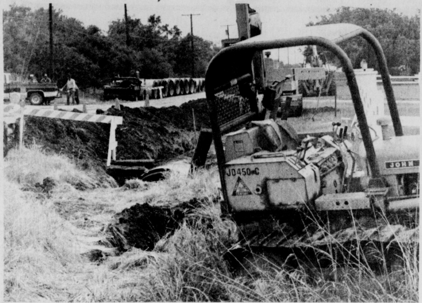
WORKMEN ABOUT READY TO CROSS JOHNSON ROAD WITH STORM DRAIN PIPE . . . street will be closed late this week or early next week.
