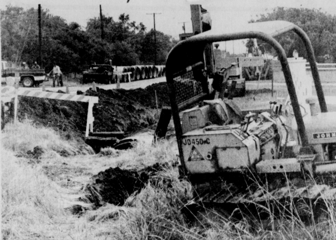
WORKMEN ABOUT READY TO CROSS JOHNSON ROAD WITH STORM DRAIN PIPE . . . street will be closed late this week or early next week.
