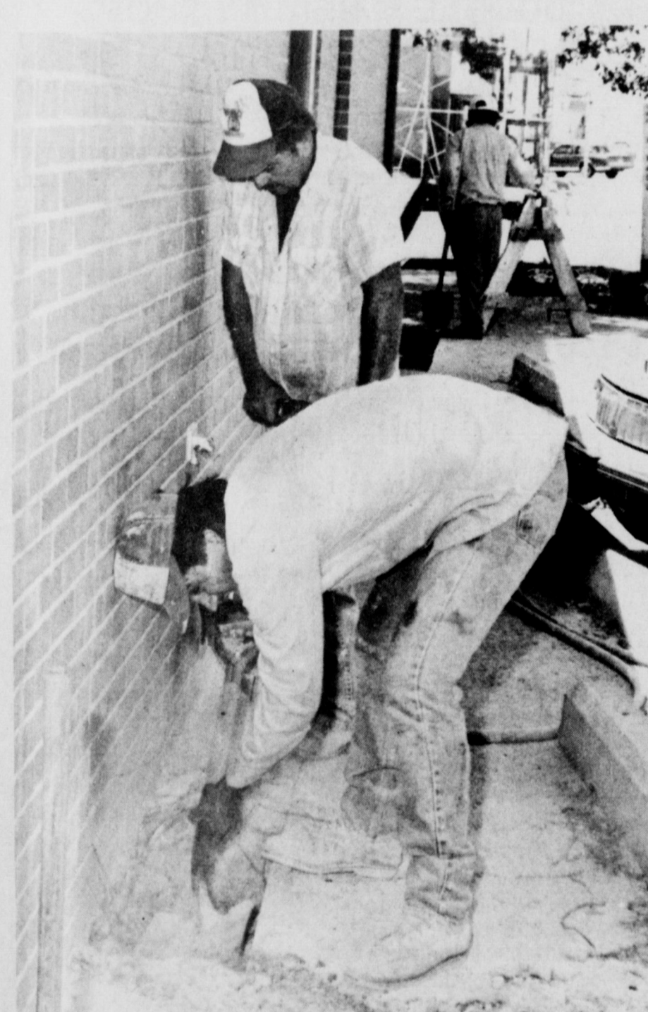
WORKERS BEGAN this week with preparations for the exterior renovation of city hall, by digging foundation holes at locations around the wall, despite the extreme heat.
