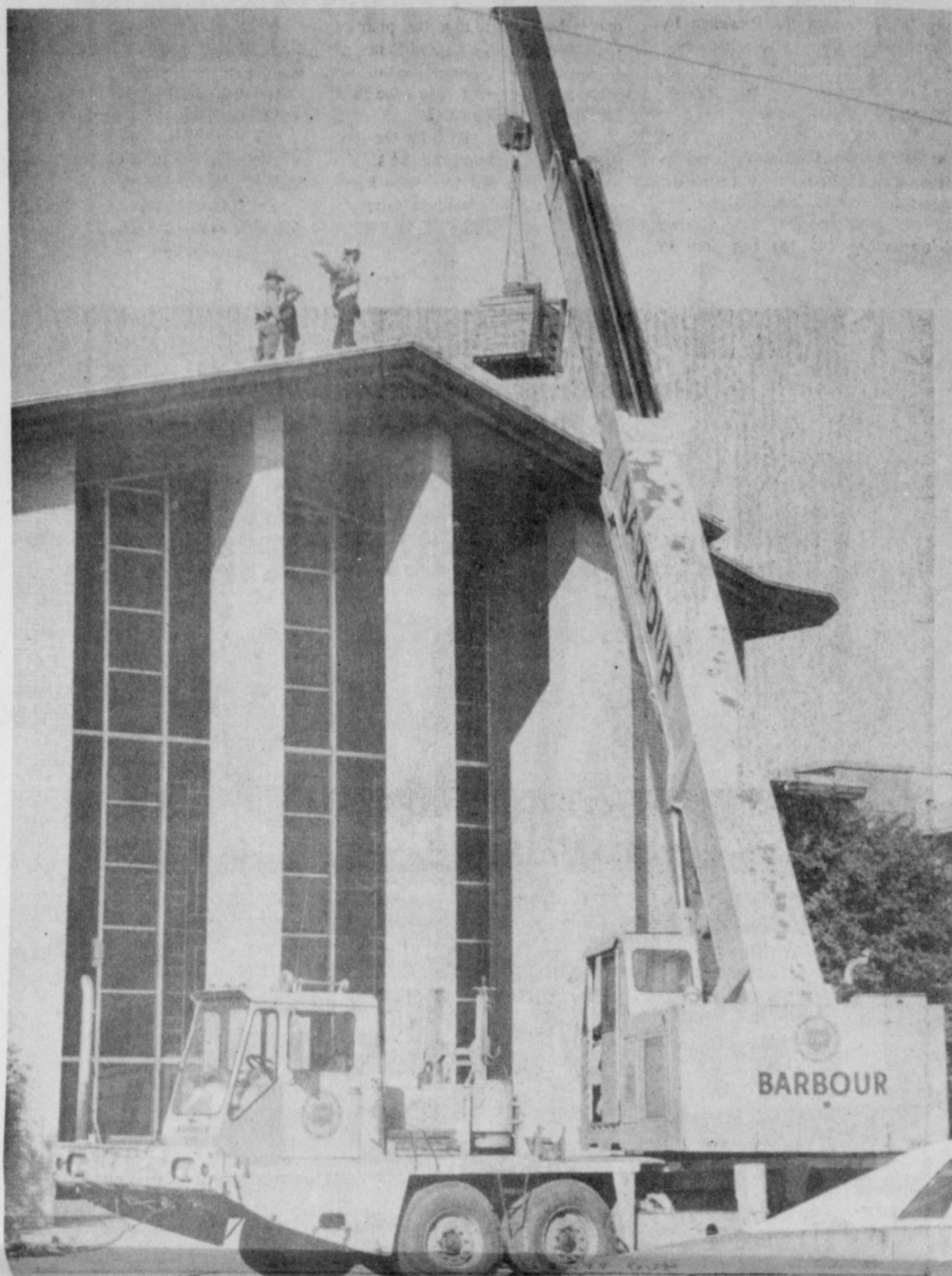
BIG JOBS require big equipment, and that's what was pressed into use Tuesday when new shingles were hoisted atop the First Baptist Church sanctuary. The project is so big that workers required more than a week to take off the old shingles.
